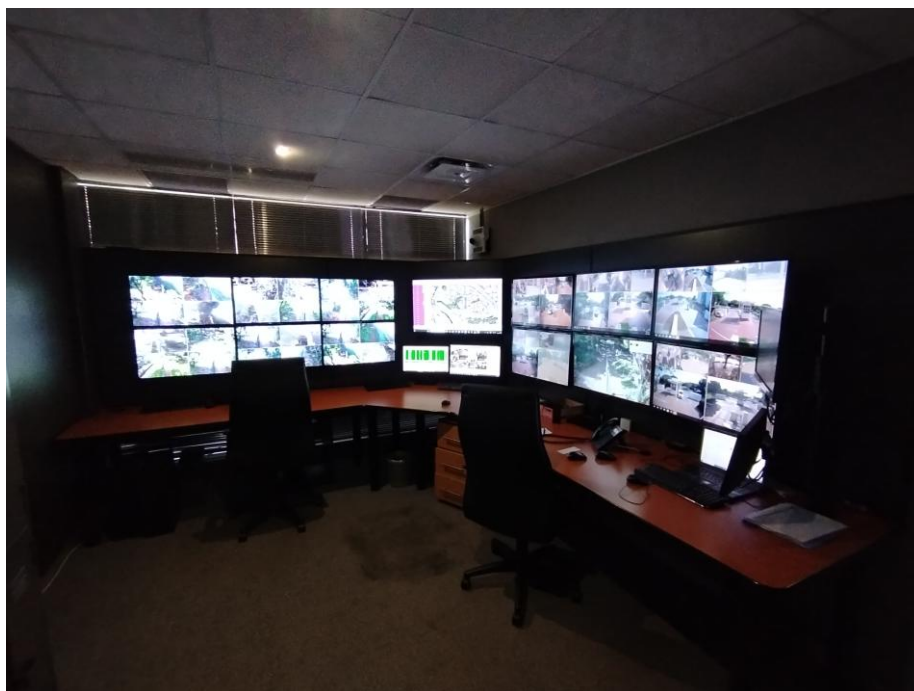
Figure 2 – Our new Control Room layout for enhanced fenceline surveillance.
