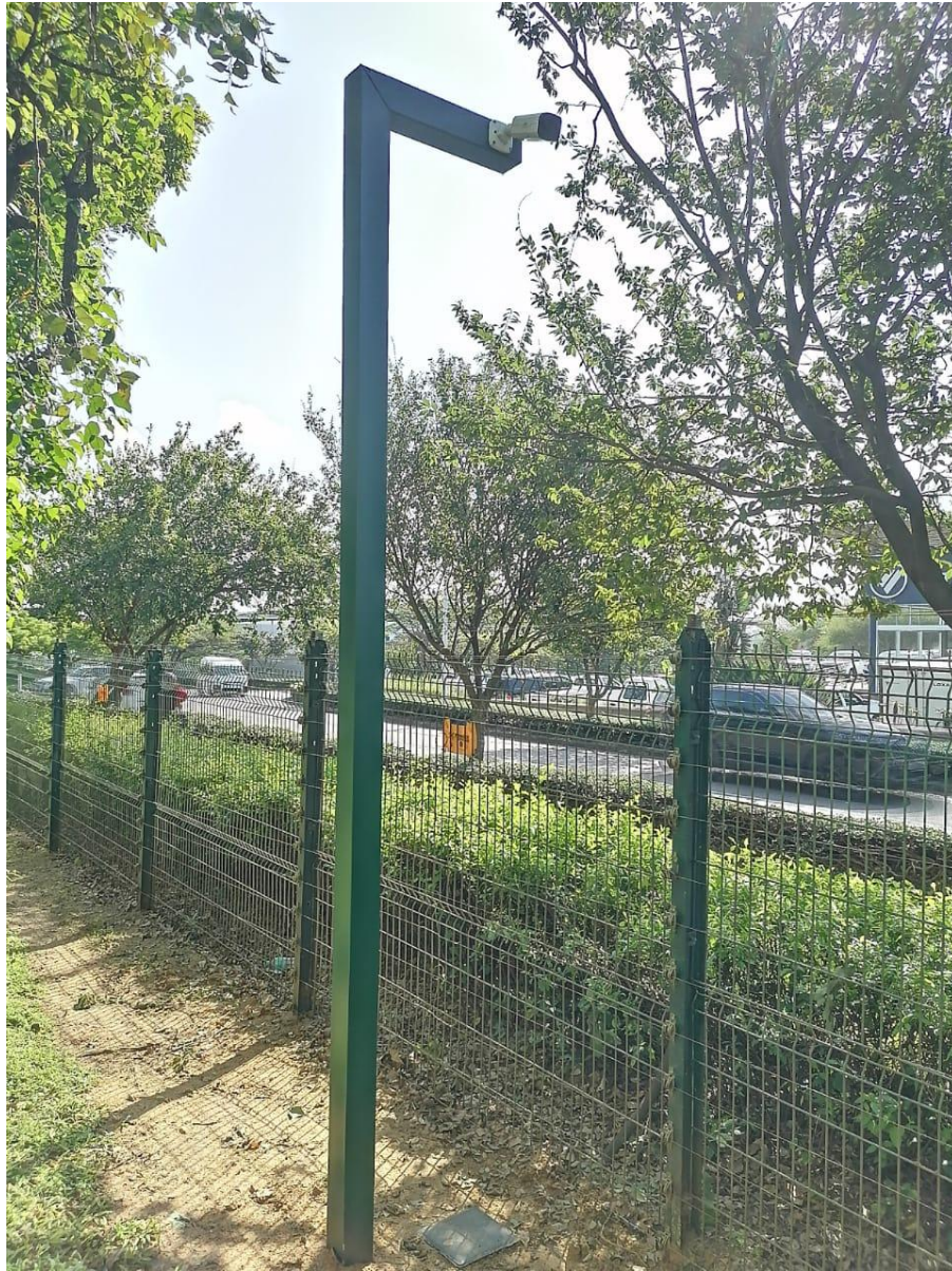
Figure 1 – An example of a new camera positioned on fenceline (Holwood Park).
